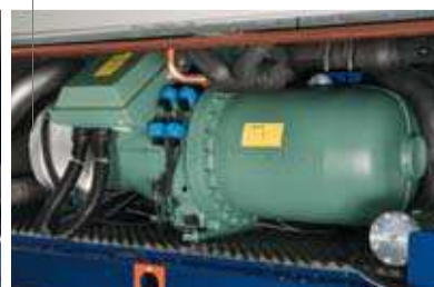
Unimpeded access to the compressors
